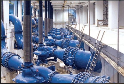
Pumps and compressors
